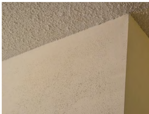
Figure 1 – Asbestos containing ceiling stipple (top of photo) and wall texture (Unit 609)
