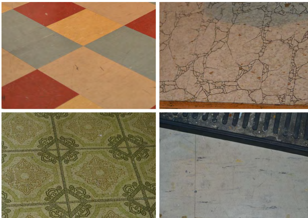
Figure 3 – ASBESTOS CONTAINING Vinyl Floor Tiles. Top left: red, green, beige, and yellow tiles from the basement bicycle room. Top right: rock pattern tiles from Unit 104. Bottom left: green pattern tiles from Unit 608. Bottom right: white speckled floor tiles from Unit 1507.
